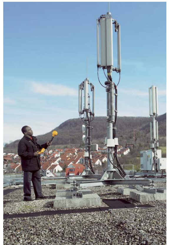
Typical site with several mobile phone antennas for GSM 900, GSM 1800 and UMTS
