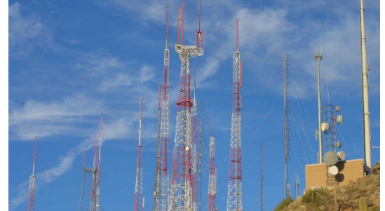
Investigating the radiation performance of antenna installations
